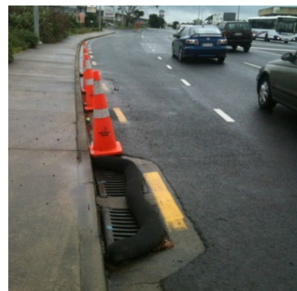
Figure 99: Installation of a silt sock to provide some protection to the catchpit
