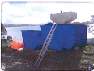
Seditrol Treatment Device in Operation in East Auckland Removing Sediment before it Discharges to the Harbour
