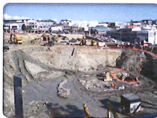
The Soho Square Development in Central Auckland where Seditrol Provided Sediment Management
