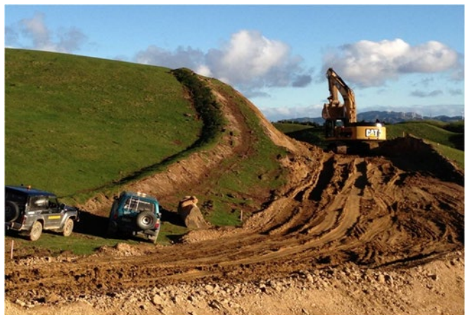
Figure 15: Clean water diversion used to isolate upper clean water flows from the works area
